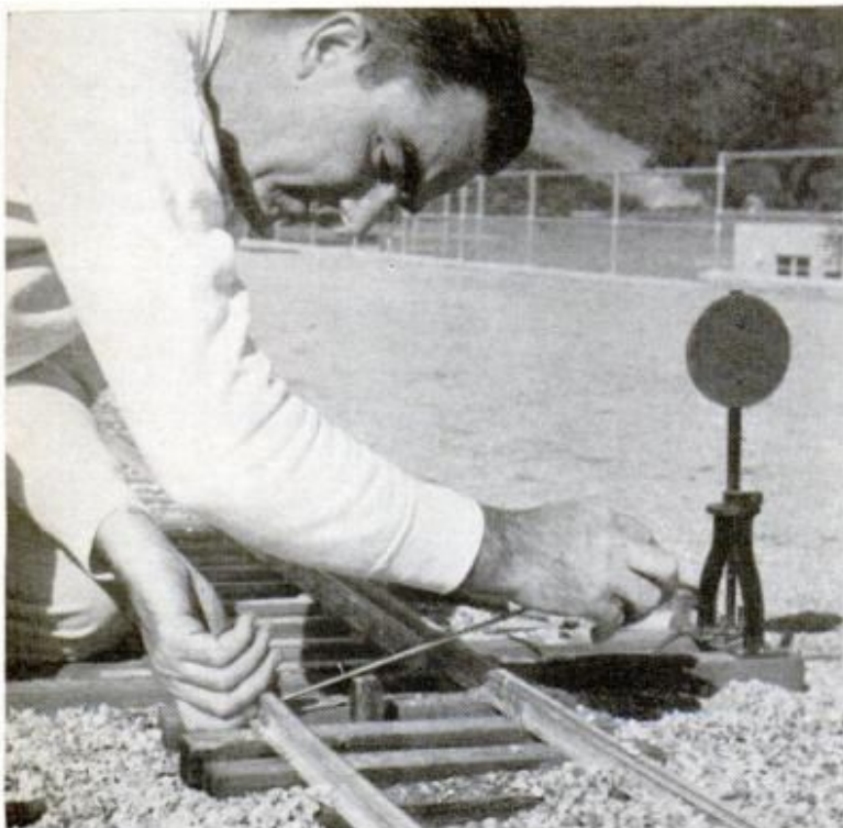
MINIATURE SWITCH is installed on 1½-inch track on Johnson's mountain. "Gandy dancers" work alternate Sundays. One club works on 1½-inch track and the other on 3-inch track, getting them ready
